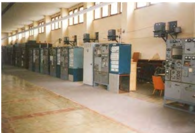
<<< Illustration 09 West side of the transmitter hall of the Funkstelle Zeesen
